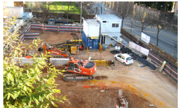
Construction of the new premises of the FLUMEN Institute at Campus Nord, UPC, Jan. 2015
